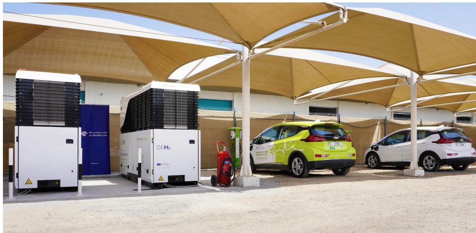
EV Charging UAE @ AI Ghandi
